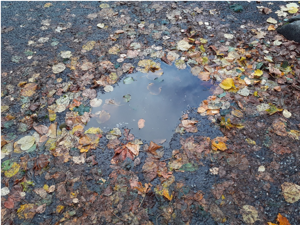
Kirkhill Square: Pothole repair needed in carpark to left
