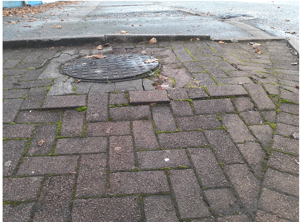
Entrance to Ardmillan Square : block and kerb repair needed at manhole cover
