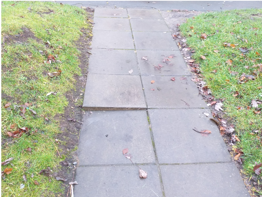
Path at side of [redacted] Sundrum Place: Slab raised in excess of 20mm Has movement when walked on
